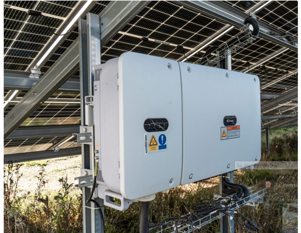
Plate 2: Typical mounting structures and string inverter
