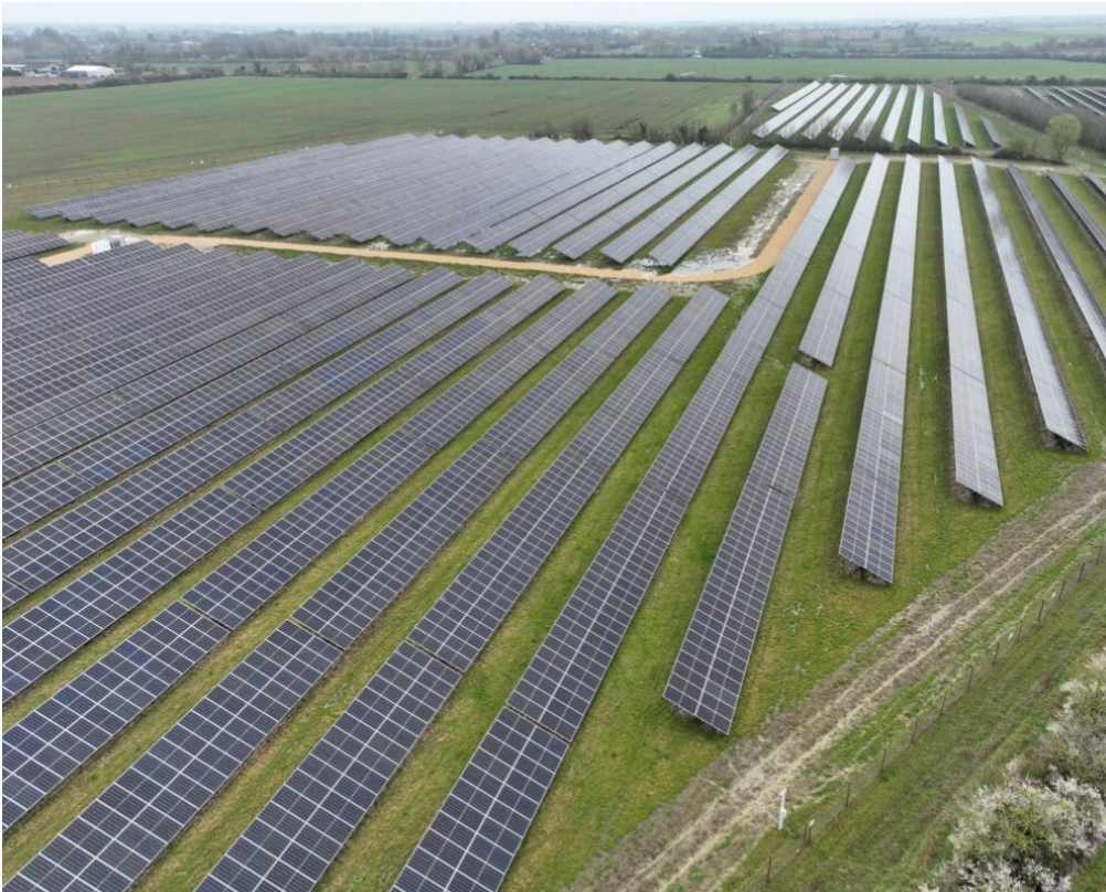
Plate 1: Typical Solar PV Panels
